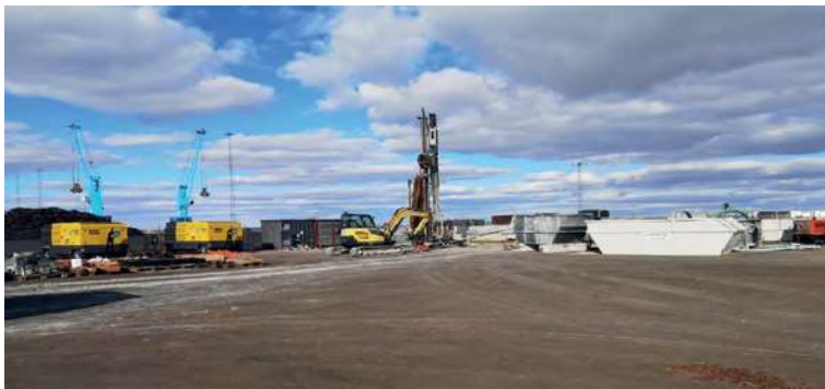
St1 Oy is drilling a deep geothermal well pilot project in Malmö, Sweden, with a Comacchio MC 900P rig
